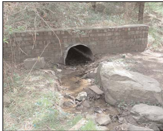
Storm-water infrastructure within the park.
