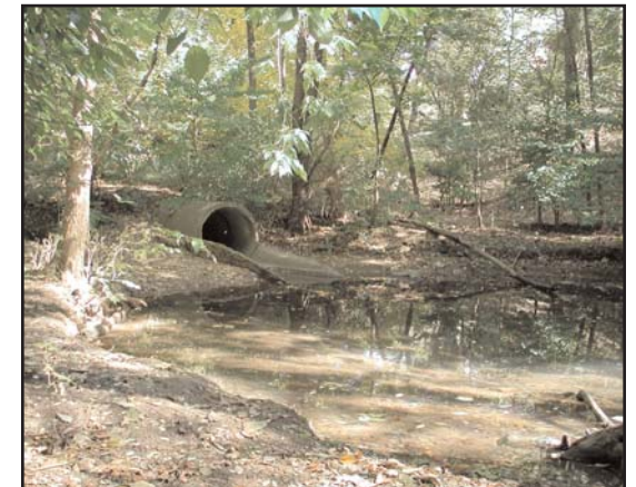
Public trails should avoid dangerous features such as this unprotected storm sewer outfall.
