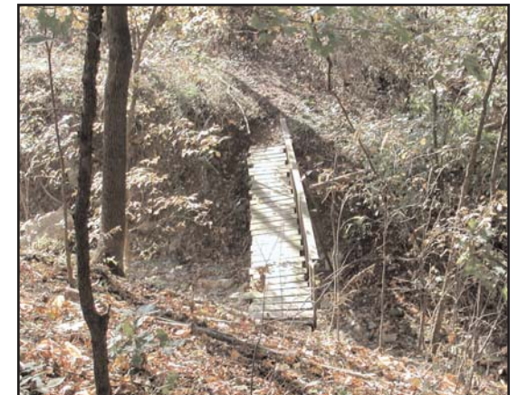
Pedestrian bridge needs to be replaced.
