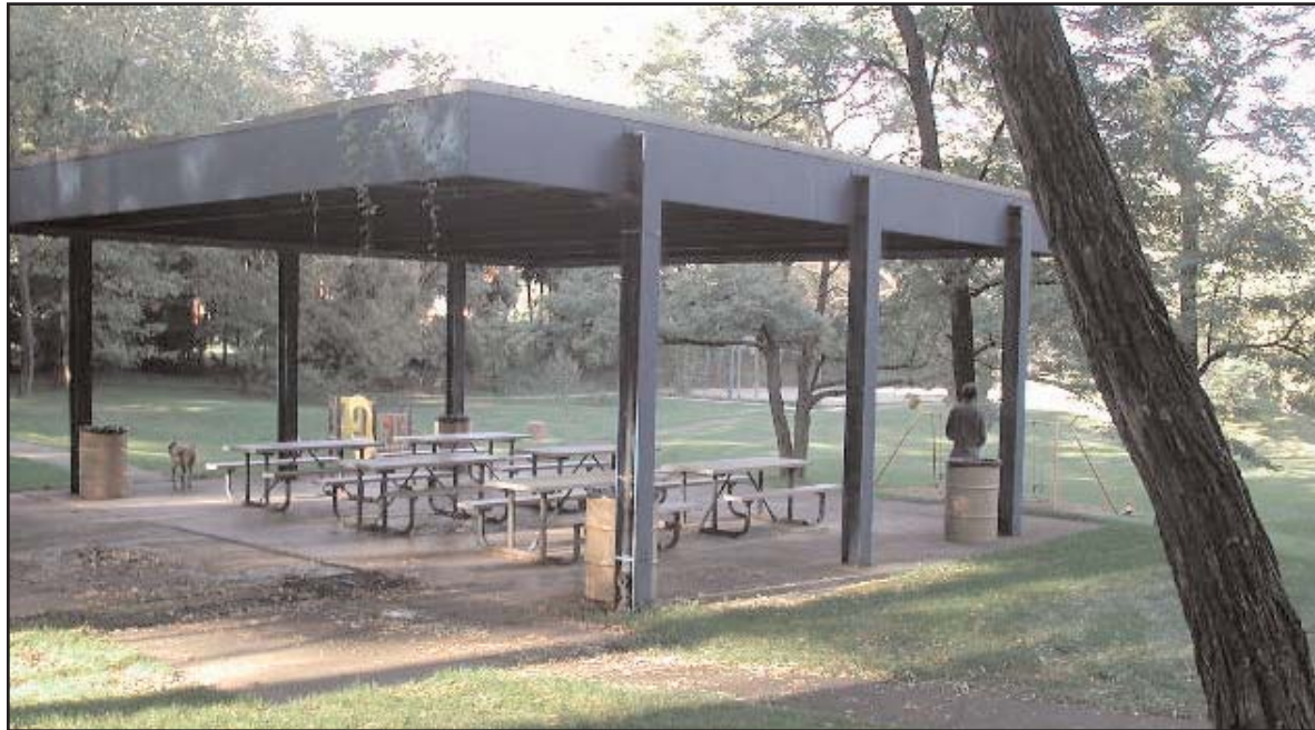
Blue pavilion is unattractive and in disrepair. A new pavilion located closer to the road would be easier to access and maintain.
