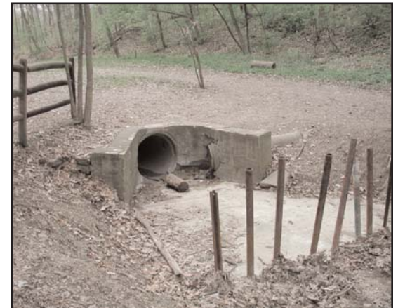
Stream conveys storm-water to this deteriorating pipe inlet.
